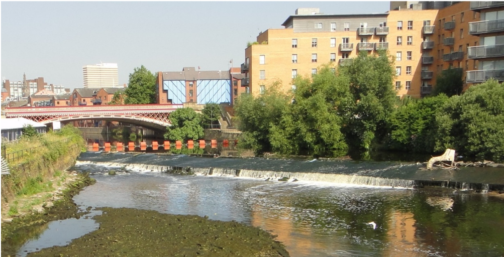
Photo 7: Leeds Dam – debris and damage to boards
