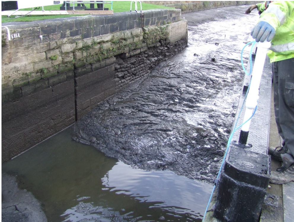
Photo 8: Masonry condition at Knostrop Quay
